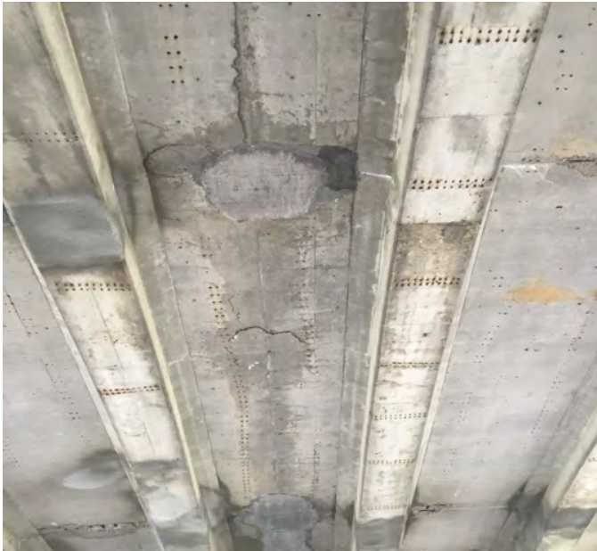
PHOTO 3 Description Span B Bay 4 exhibits approximately 10 SFT of delamination that needs removed over traffic lanes.
