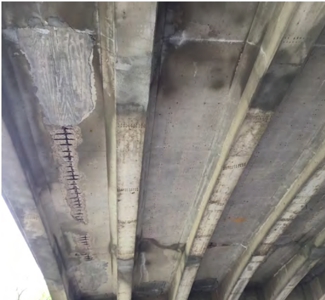
PHOTO 4 Description Underside Span B exhibits approximately 80 SFT of spalling with exposed reinforcement.
