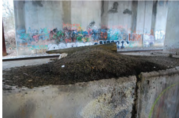
Guano location 1: Guano on concrete wall of pier 3 between columns - 12/27/2021
