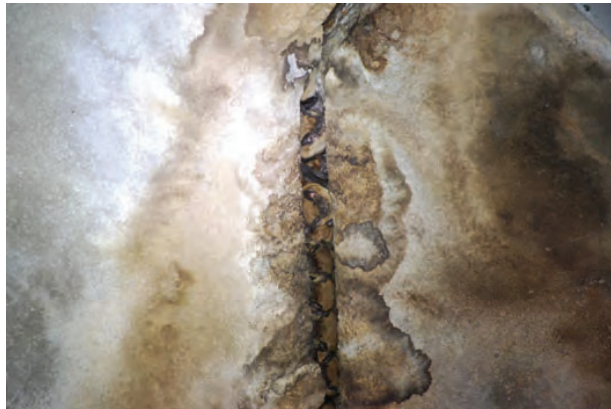
Bat location B: Big brown bats (30+) in expansion joint gap above pier 3 between center columns - 9/2/2021
