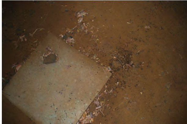
Guano location 6: Guano on dirt slope wall east of pier 3 under beam 8 - 12/27/2021
