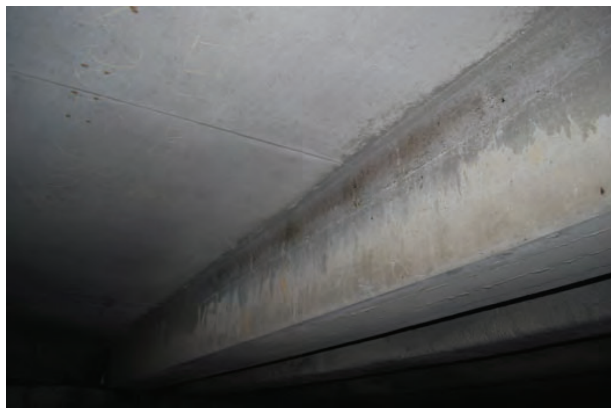
Staining location 7: Staining on north face of beam 5 - 12/27/2021
