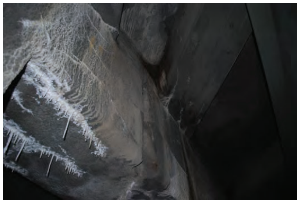
Staining location 5: Staining in corner at top of pier 3 between center columns - 9/2/2021
