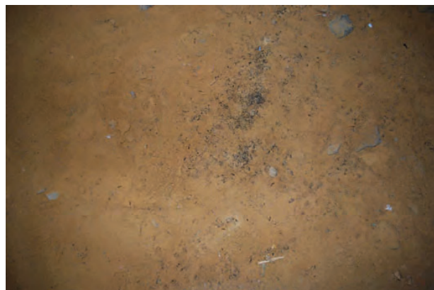
Guano location 5: Guano on dirt slope wall east of pier 3 under beam 5 - 12/27/2021
