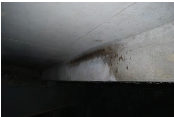
Staining location 6: Staining on south face of beam 4 - 12/27/2021
