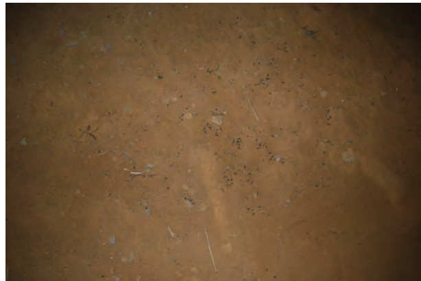
Guano location 3: Guano on dirt slope wall east of pier 3 under beam 3 - 12/27/2021
