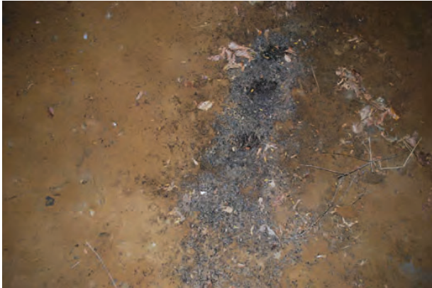
Guano location 6: Guano on dirt slope wall east of pier 3 under beam 7 - 12/27/2021
