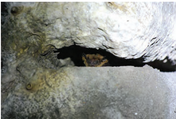
Bat location C: Big brown bat in expansion joint crevice above pier 3 center columns on east side of railroad - 12/27/2021
