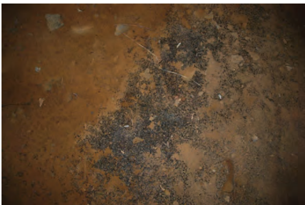
Guano location 4: Guano on dirt slope wall east of pier 3 under beam 4 - 12/27/2021
