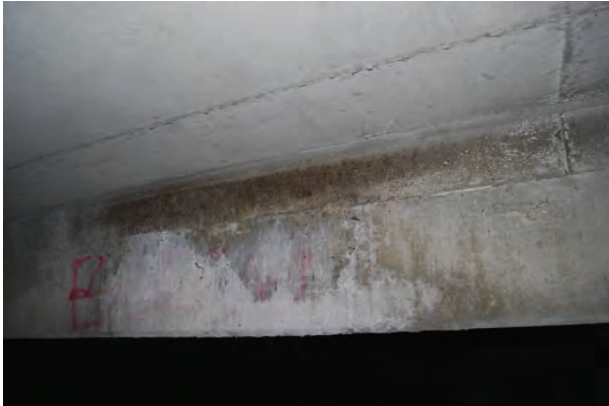
Staining location 8: Staining on north face of beam 7 - 12/27/2021
