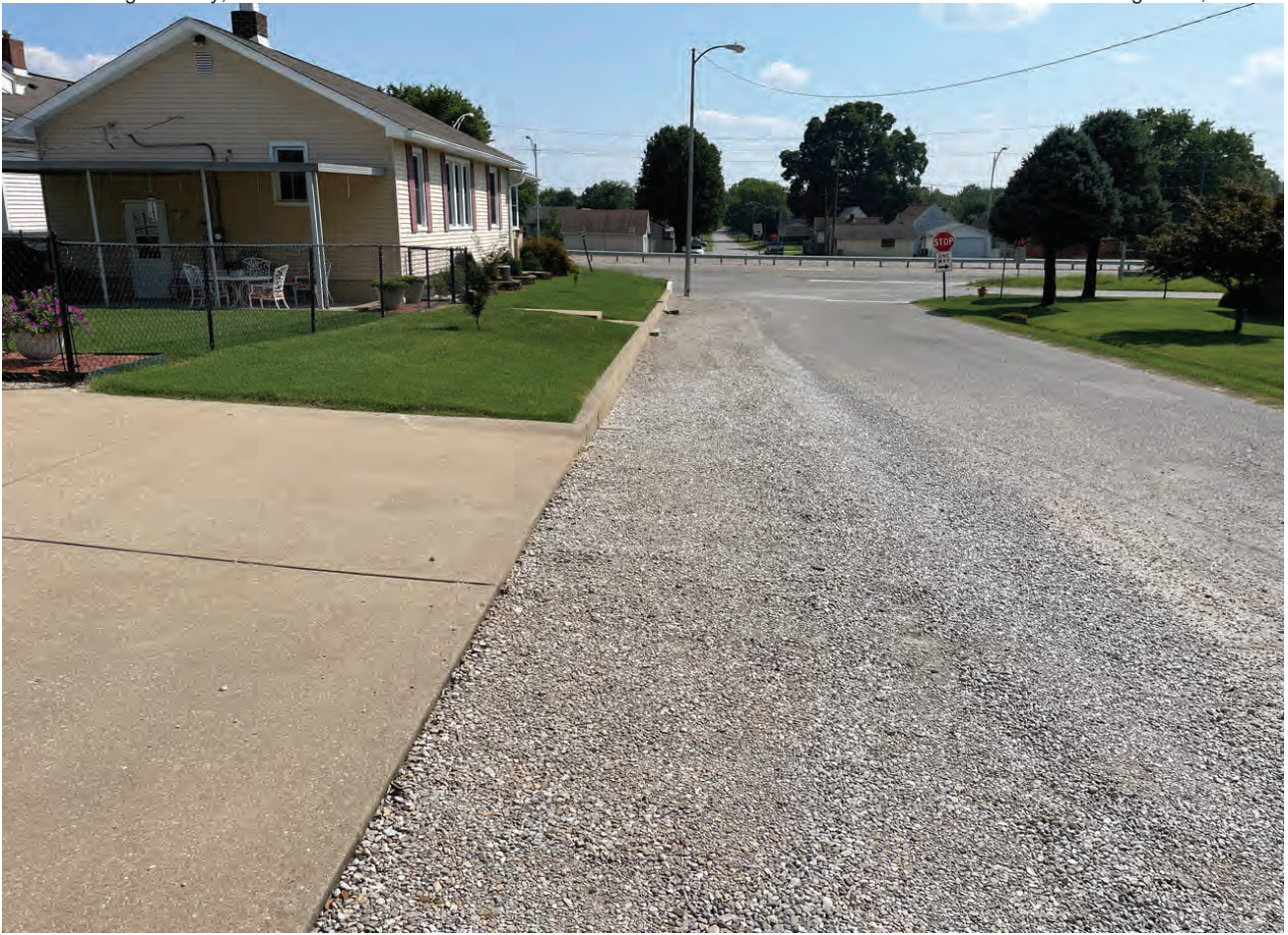
11. Facing south along Ingle Avenue towards Corbierre Avenue intersection, north of SR 62.
